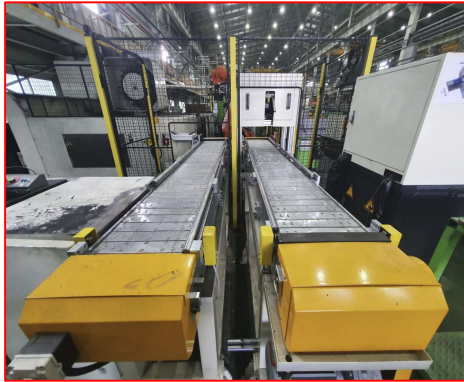
< Steel transfer conveyor >
